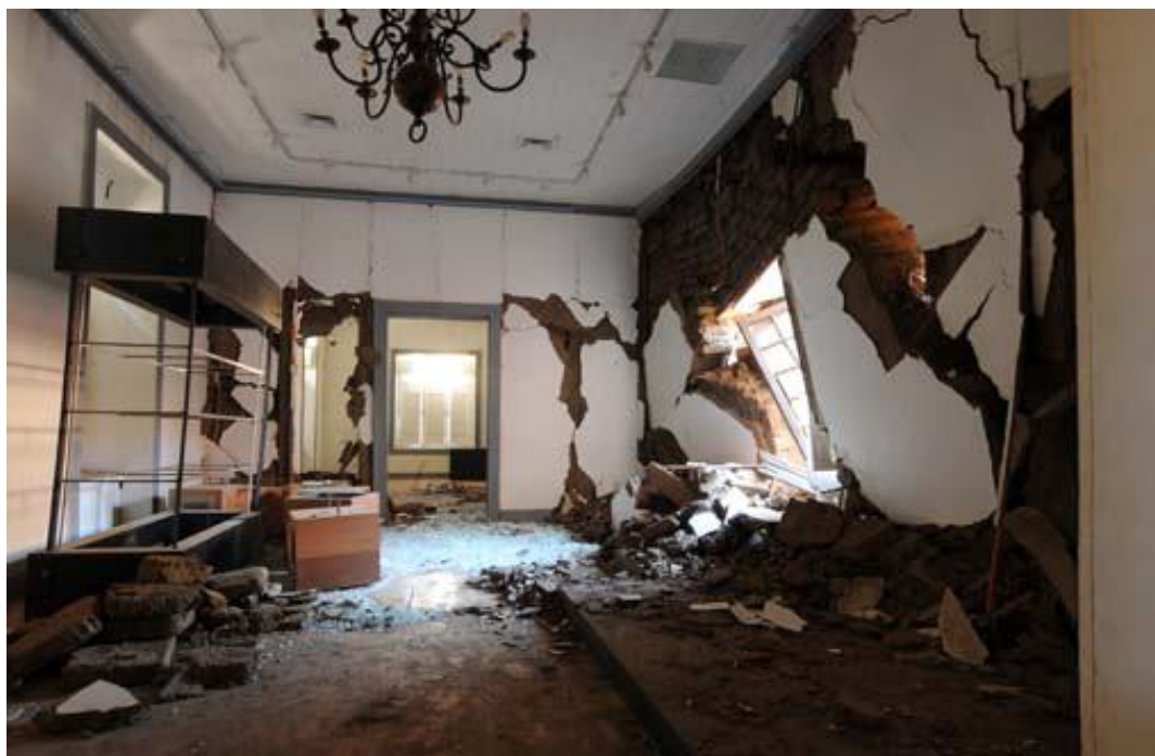
Εικόνα 15: Earthquake damage at the Museo de Bellas Artes de Talca, Chile. Photo: Jorge Sacaan Riadi( πηγή: http://blogs.getty.edu/iris/update-on-the-earthquake-in-chile/ )
