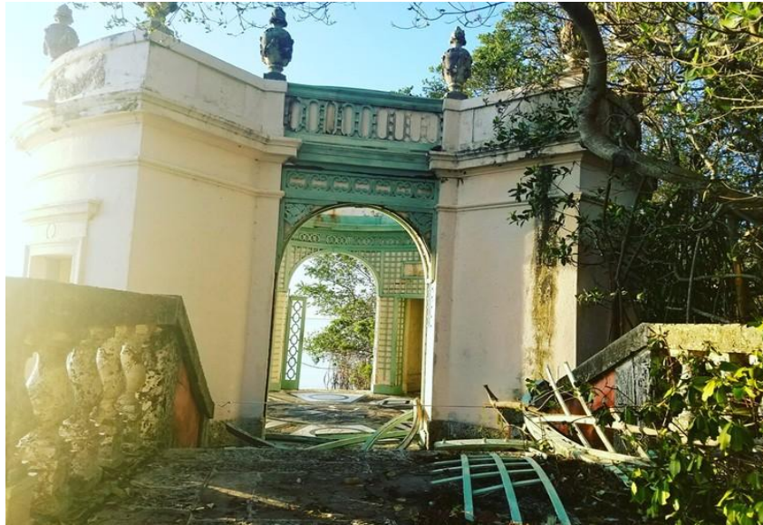
Εικόνα 12: Vizcaya's Tea House lost its wood trellis roof during Irma. (πηγή: https://www.miaminewtimes.com/arts/volunteers-at-vizcaya-get-free-family-pass-9670892 )
