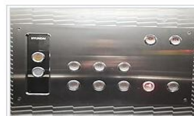
Elevator buttons with Braille markings
